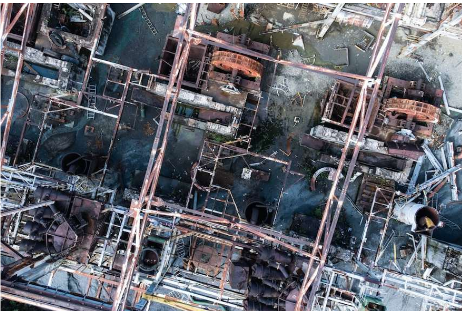
Families live among the skeleton of the mine's concentrator, which can be traced back to a mining operation in the 1970s and 1980s. (ABC News: Tim Swanston)
